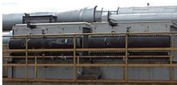
Fig. 6 Outer appearance of a heat-exchanger that was used as an object of a demonstration test and was actually operated for production.
